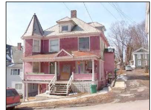
Above (top to bottom): Poorly maintained rental apartments at the base of Leonard Street; view of back yards of rentals; and poorly maintained rental on Leonard Street. These structures have major deficiencies .
