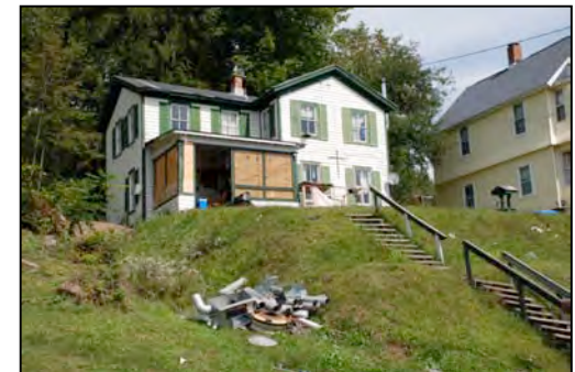
Above (top to bottom): Poorly maintained housing on East Main Street some involving single-family homes converted to multi-unit apartments. Houses with major deficiencies such as poorly maintained steps, boarded up windows, peeling paint or other deferred maintenance detract from surrounding property values. These units stand in sharp contrast to beautifully maintained homes along this street.
