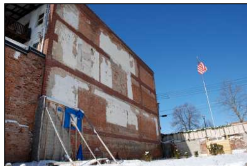
Above: Temporary supports provided to stabilize wall of building adjacent to the Property. The construction of the Gateway Building will help to stabilize adjacent buildings along Front Street.
