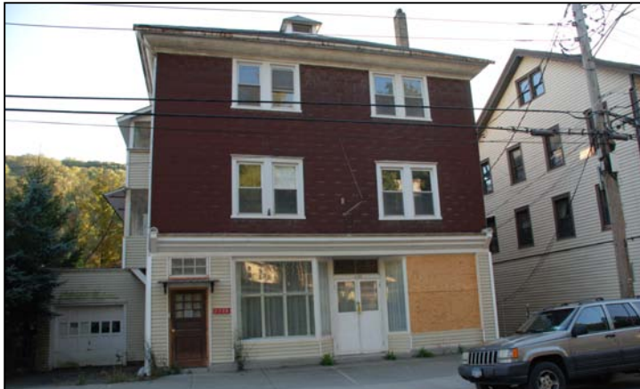
Above: This mixed-use building at 1130 Main Street has a hipped roof, decorative lower cornice above the storefront, recessed entry and large display windows. The renovation of this storefront should be limited to needed repairs, painting and replacement of the storefront glass.
