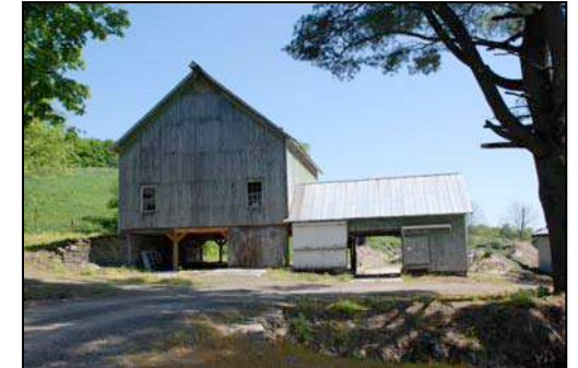
Above (top to bottom): Barn and silos in good repair along NYS Route 51; interior view of restoration and reconstruction of the Morehouse main barn; and recently restored barn on the Morehouse Farmstead. As long as the frame, foundation and roof are structurally sound – most barns can be restored. This Plan supports efforts by local landowners to restore historic barns.
