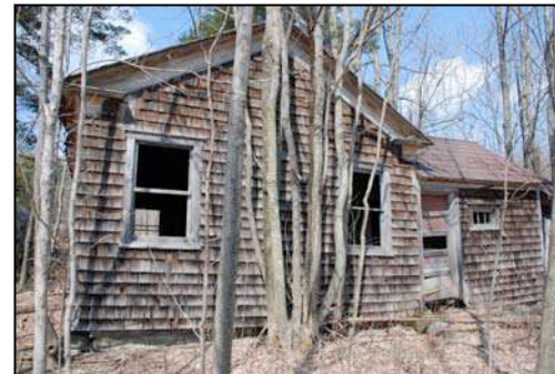
Above: School District #12 - Naylor's Corners Schoolhouse at the corner of CR 12 and Gross Road. Despite years of neglect, the schoolhouse is remarkably still in tact. However, without some immediate efforts to stabilize the structure and remove trees that are growing in close proximity to the foundation this building will soon be lost to the elements.
