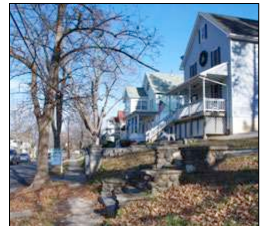
Above (top to bottom): Residential street with sidewalk system in good condition; ADA compliant ramp at corner of NYS Route 52 and Elm Street; and view of bluestone sidewalks, which need to be re reset, repaired or replace due to tree uprooting sidewalk segments.
